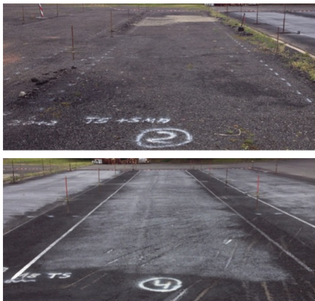
Figure 7: Examples for prepared base surfaces (top picture: gravel base, bottom picture: asphalt base)
