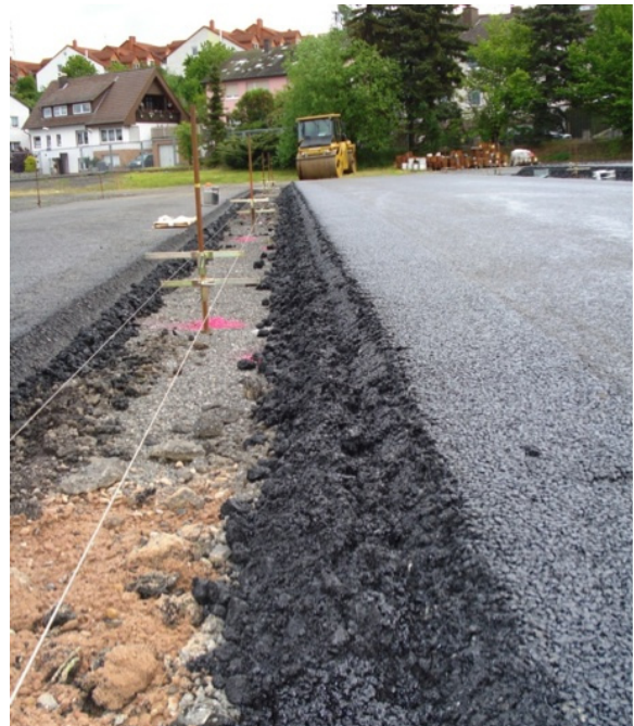
Figure 12: Unsatisfactory appearance of edges on thick compact asphalt packages (right) vs. typically shaped edges on reference layer with a thickness of 12 cm (left)
