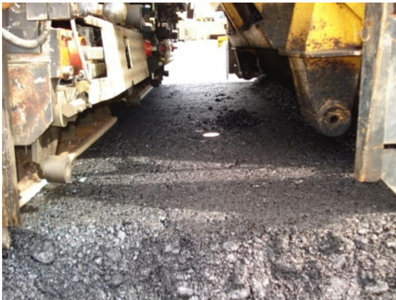
Figure 9: Surface of combined binder/base course on testing ground 3 (mod. compact asphalt 22+2 cm) in front of the wearing course screed
