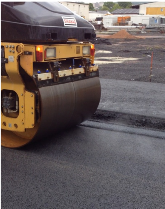
Figure 11: Instability of edge regions under dynamic roller load on thick compact asphalt packages
